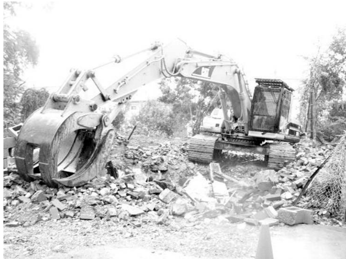
Wrecking havoc: The city of Philadelphia dedicates almost all of its money earmarked for "affordable housing" to bulldoze homes.
